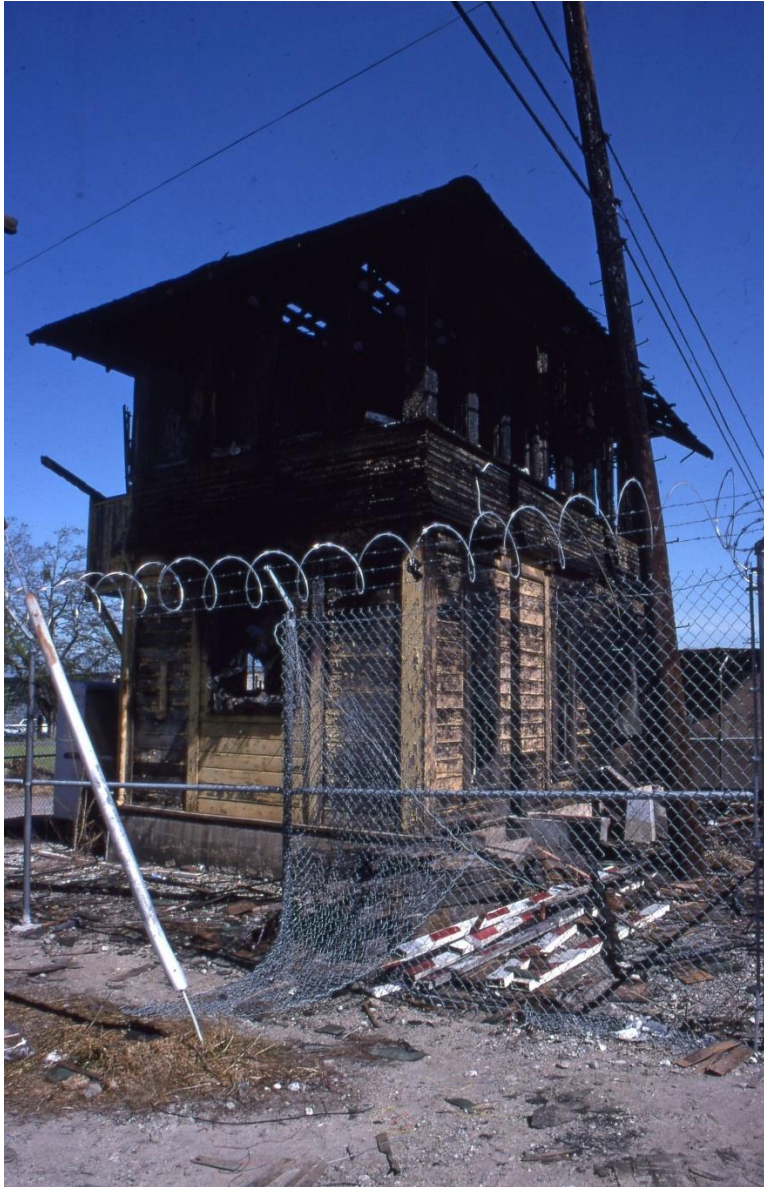
Figure 6: Southern Pacific Switching Tower Following Fire (photo courtesy of applicant)
