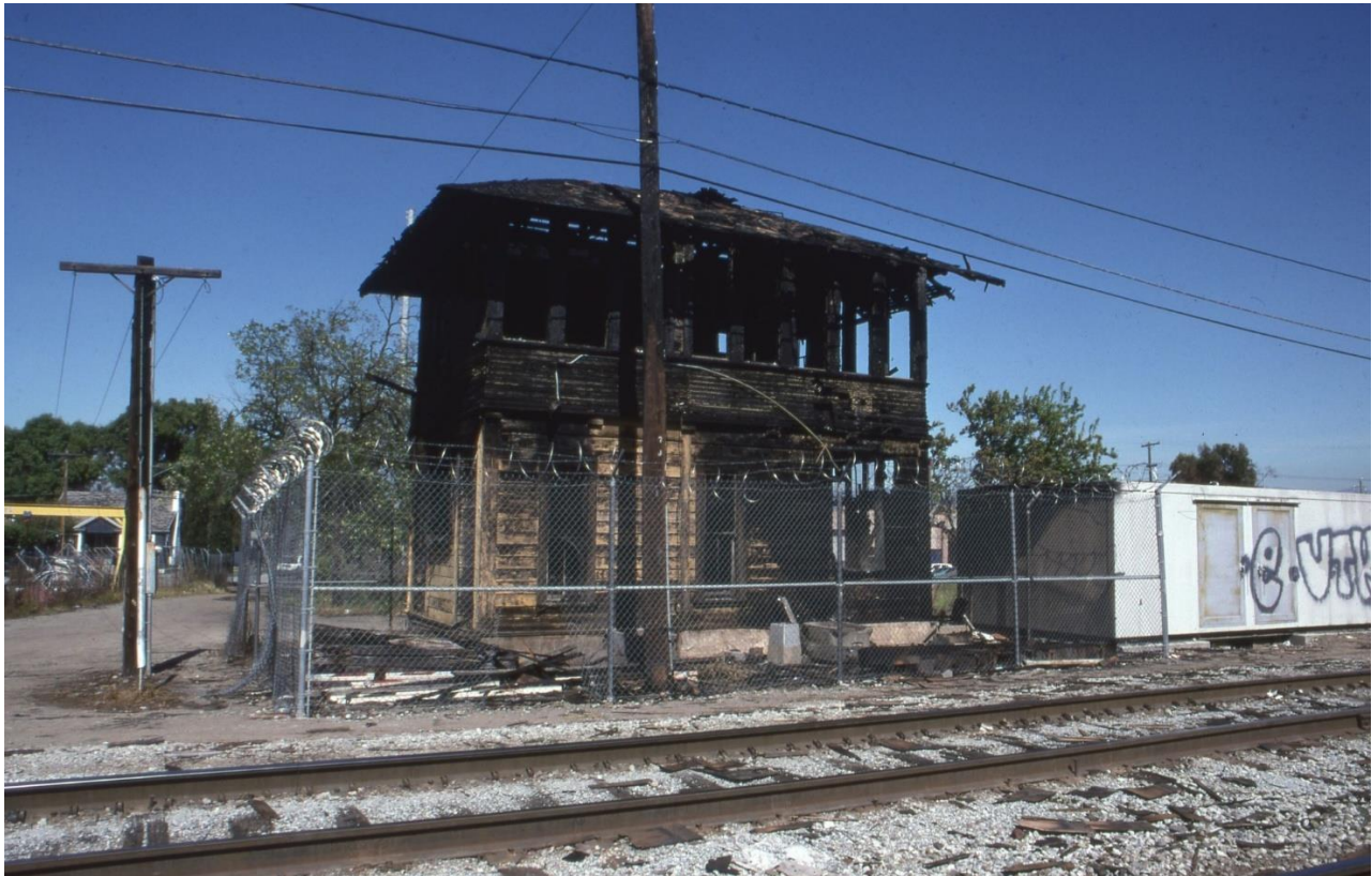
Figure 5: Southern Pacific Switching Tower Following Fire (photo courtesy of applicant)
