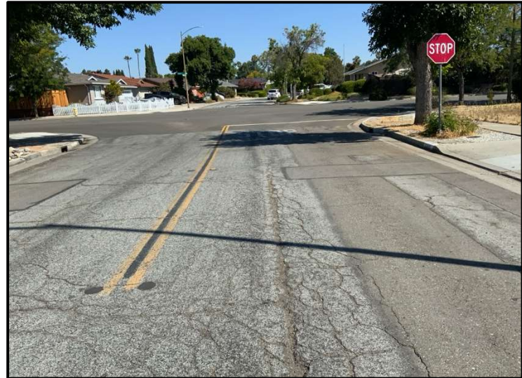
Failed (Below PCI 25) – Tandra Av: PCI 23
