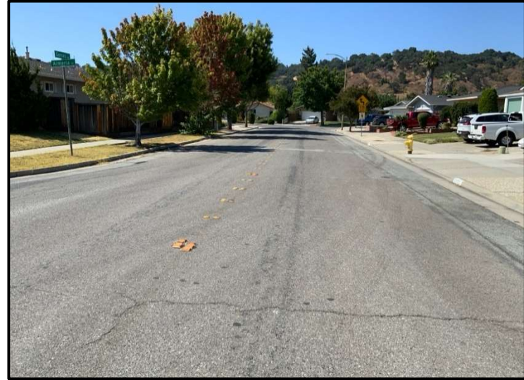
Fair (PCI 69 to 50) – Avalani Av: PCI 59
