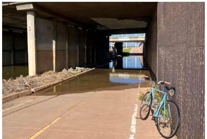
Flooding of the GRT underpass at Highway 237. Credit: Ray Hosler
