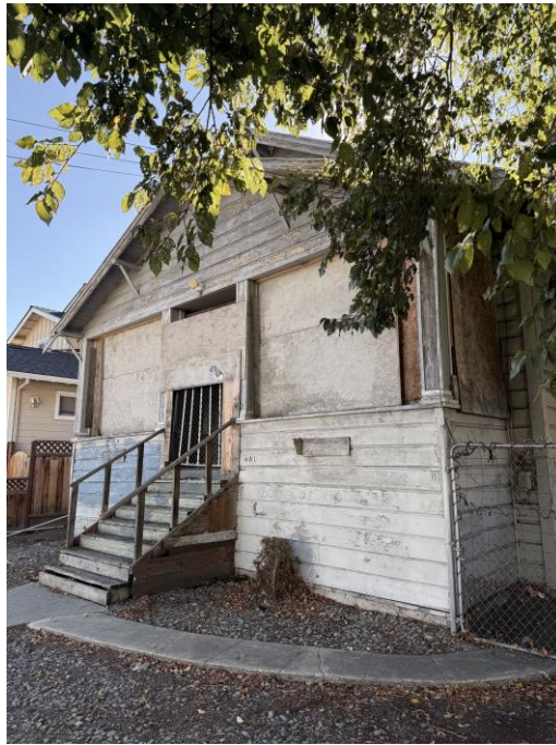
681 N 5 th Street – historic property in blighted condition (Photo taken October 27 th 2025)
