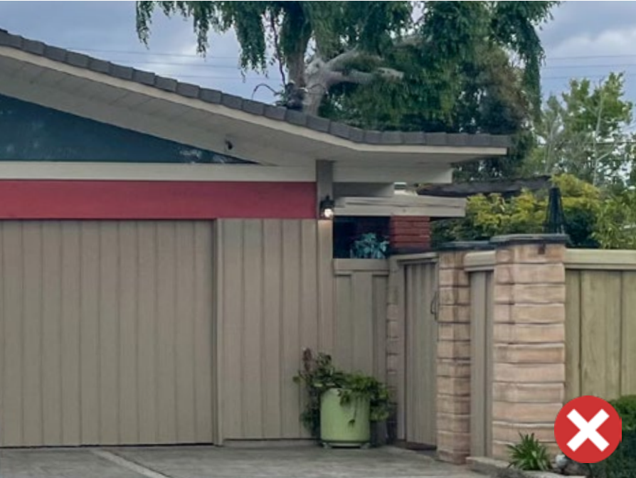
Figure 11: Concrete tile roofing is prohibited.
