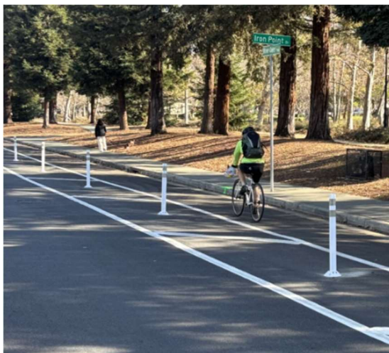
Right: In-progress bikeway on River Oaks Parkway constructed using one-time grant funds.
