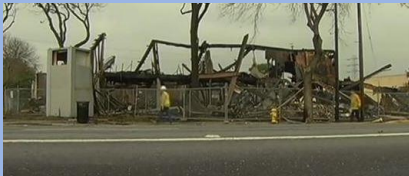
KNTV Building CA Register Eligible (Destroyed by fire 2014)
