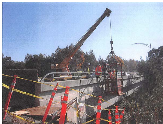
Start of installation of pipe roller hangers to hold 12" epoxy lined DIP pipe.
