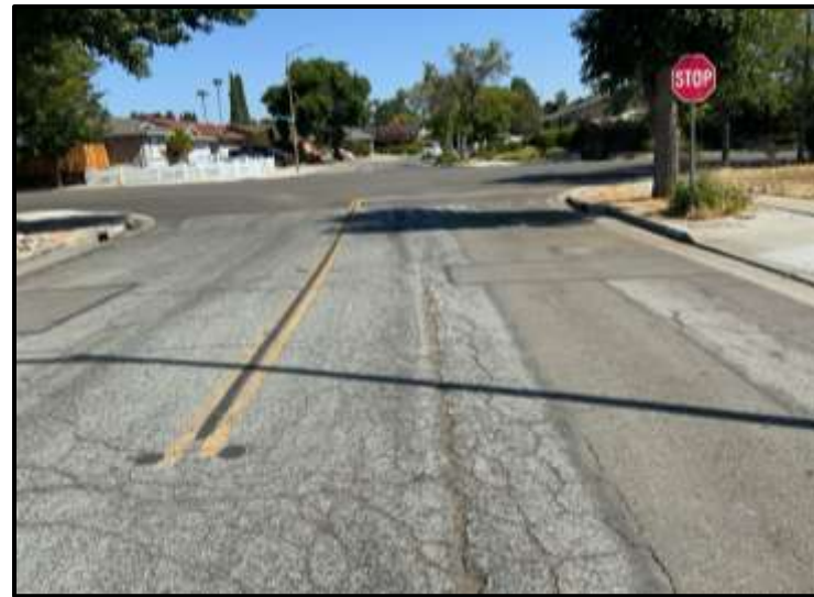
Failed (Below PCI 25) – Tandra Av: PCI 23
