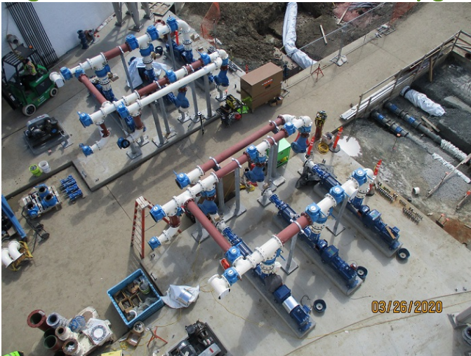
Figure 9: The upgraded foam suppression and withdrawal pumps and visible piping for thermophilic Digesters 5 and 7.
