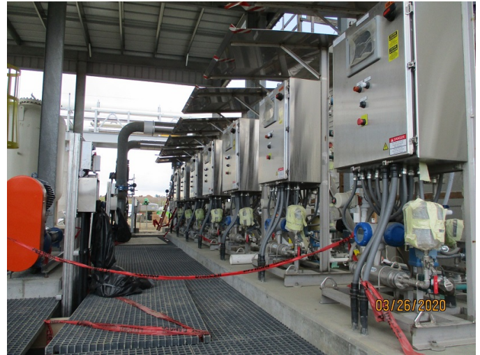
Figure 10: The automated polymer blending system will feed polymer to the blended sludge prior to entering the dissolved air flotation thickener tanks.
