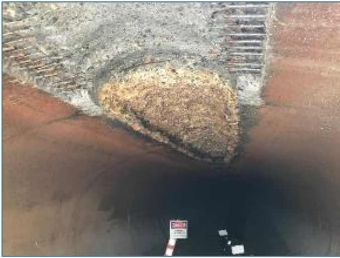
Figure 3: Rebar degradation of 96-inch SES pipeline
