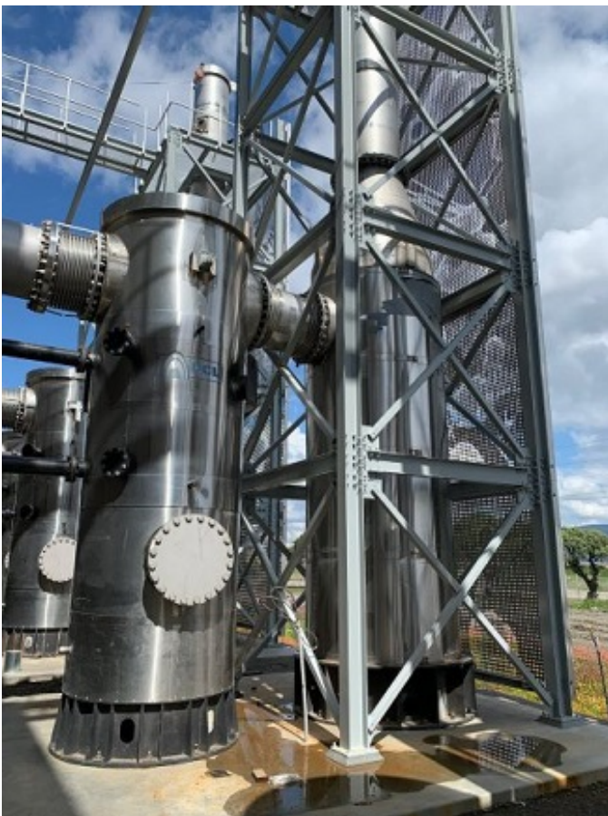
Figure 8: The new engine generators' high exhaust heat is used to produce hot water, which is then used to provide heat to the digesters and other facilities. The exhaust gas is cleaned through a treatment system before being discharged through the exhaust stacks.
