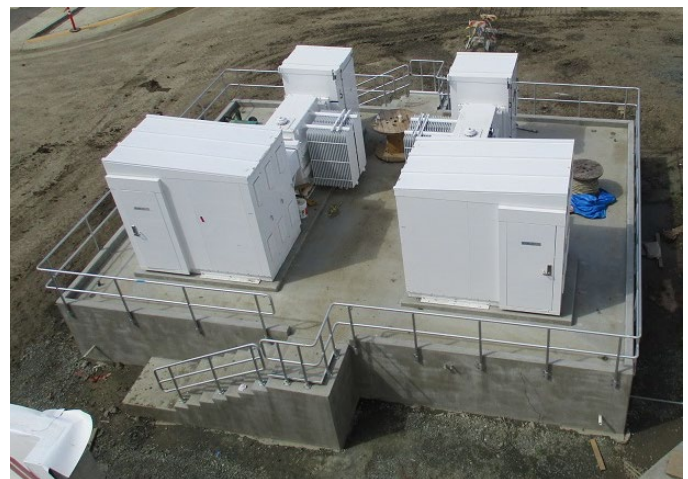
Figure 12: The new electricity load center at 5th and Center Streets will reduce the grid voltage to power the digester equipment.
