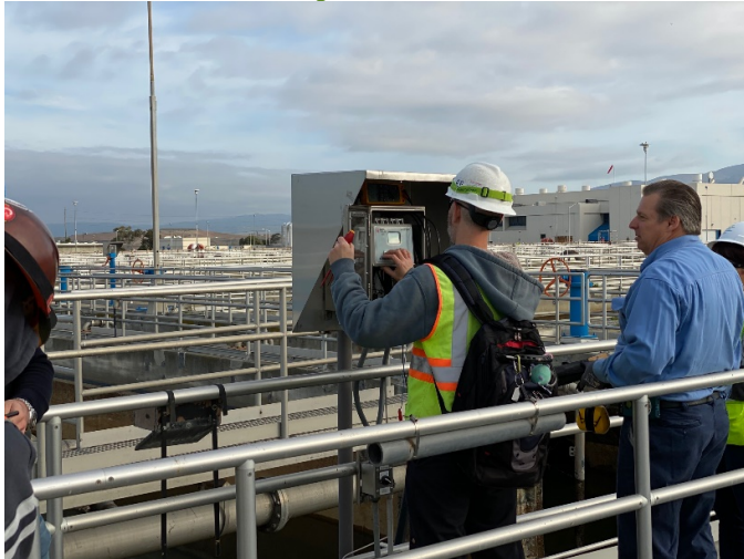
Figure 4: The contractor performs electrical instrumentation adjustments and verifies readings with an existing distributed control system (DCS) node.
