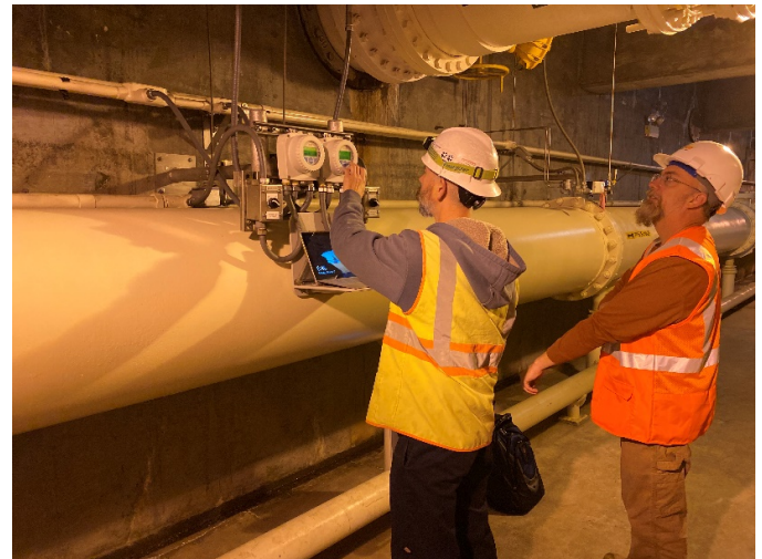
Figure 5: The contractor verifies a new DCS node located in one of the many tunnels during functional testing.
