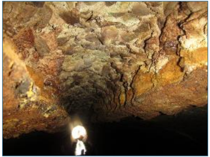
Figure 4: Crown corrosion of 87 by 136-inch SES pipeline
