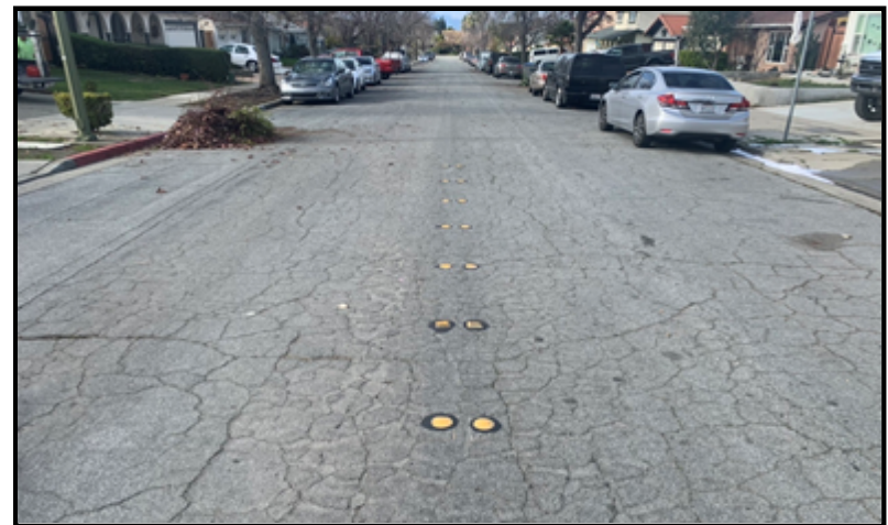
Failed (Below PCI 25) – Trebol Ln: PCI 24
