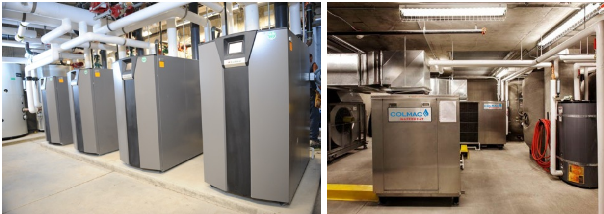
Figure 2: Central gas water heating system (left) and central heat pump water heating system (right).
