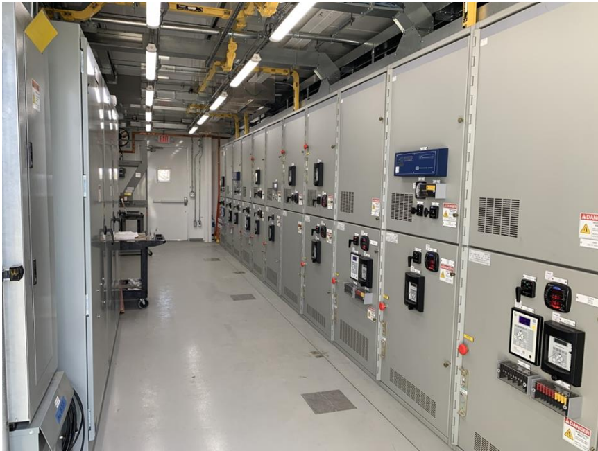
■ Interior of Switchgear enclosure
