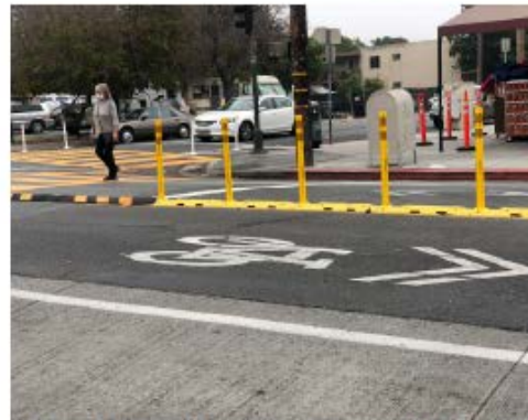
Hardened Centerline: Prevents turning vehicles from crossing centerline, resulting in slower turn speeds.
