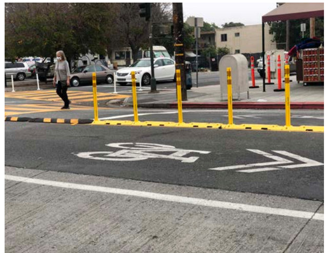
Hardened Centerline: Prevents turning vehicles from crossing centerline, resulting in slower turn speeds.
