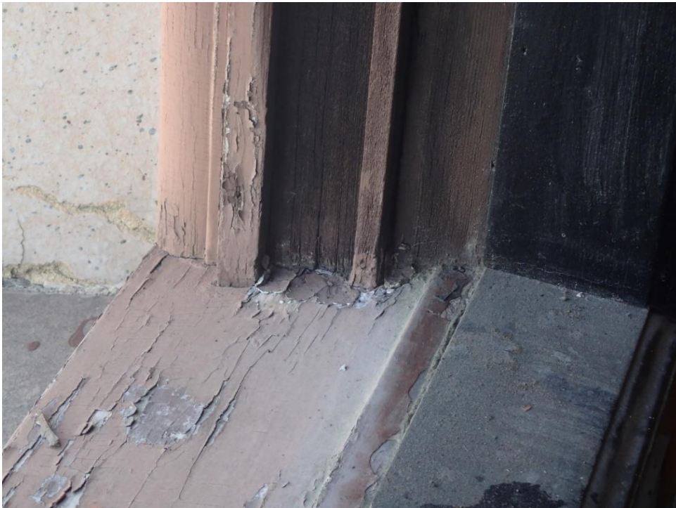
Typical deteriorated double-hung window sill and side channels
