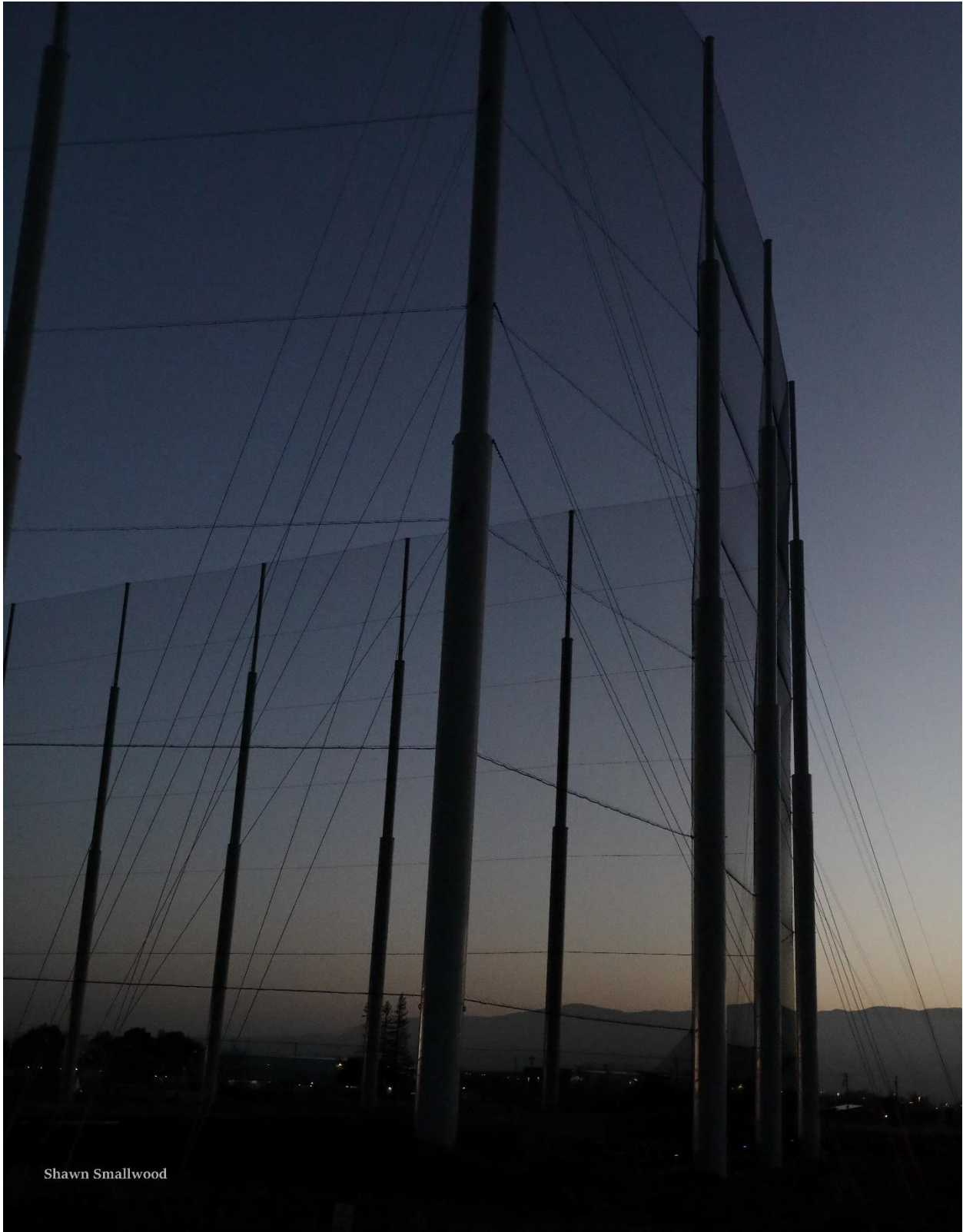
Photo 29. The TopGolf net viewed towards the glow of the rising sun at 06:42 hours, 1 April 2022. Note that the net would be less visible when viewed from the north or east. Also note that the guy cables are unmarked, and no markers are on the net.
