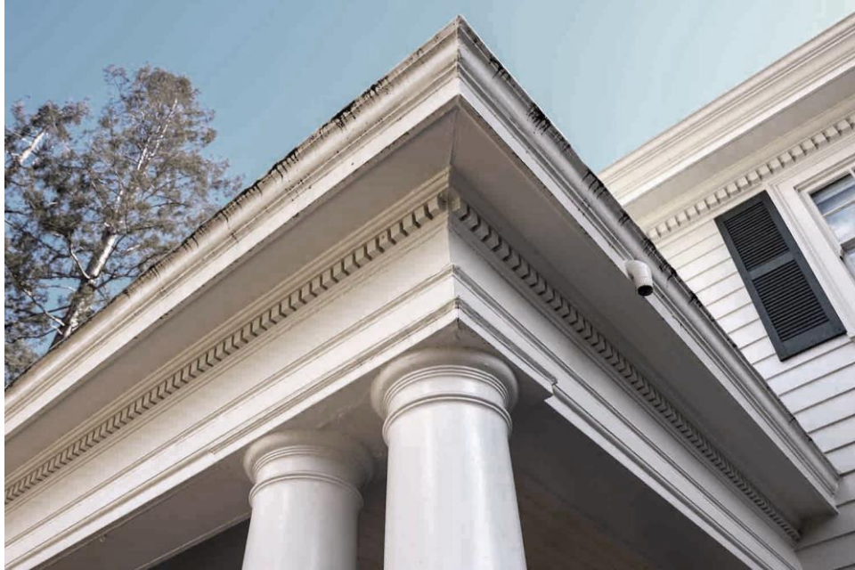
Closeup of original dentil molding under the eaves of the front porch and upper roof.
