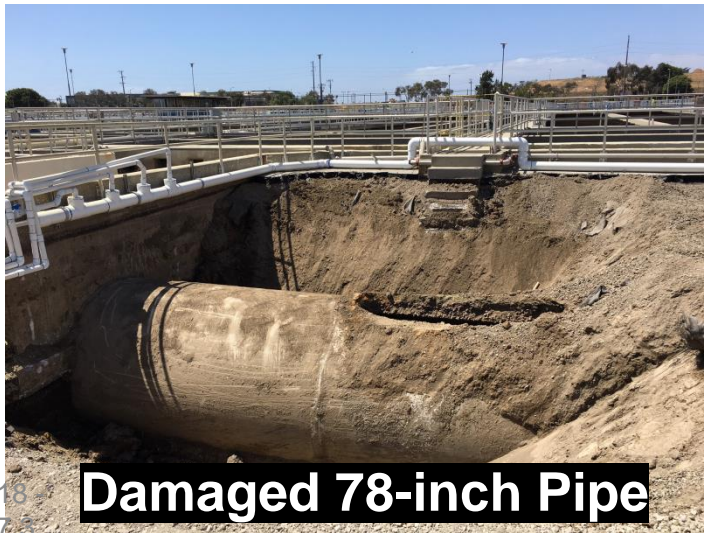
Temp. Pumping System
