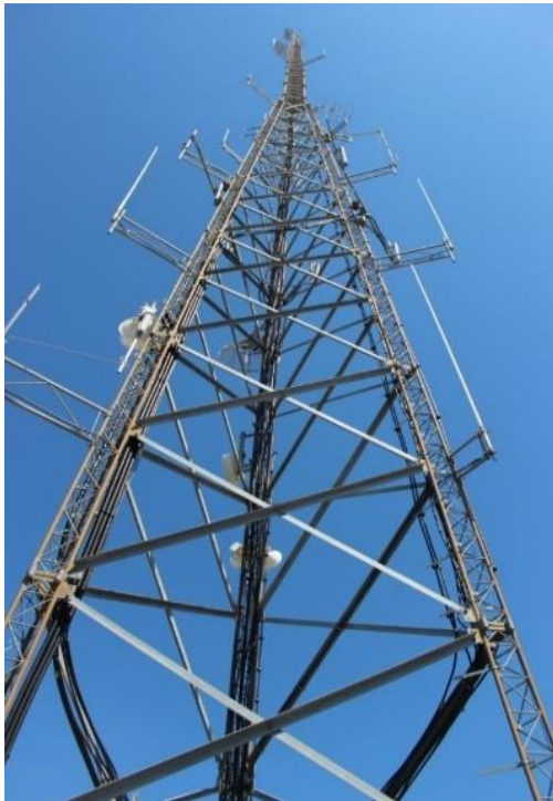
Transmitter Antennae at Coyote Peak
