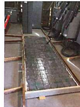
*PAC Electrical System Upgrade
