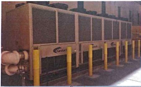
* Civic Auditorium Air Conditioning
