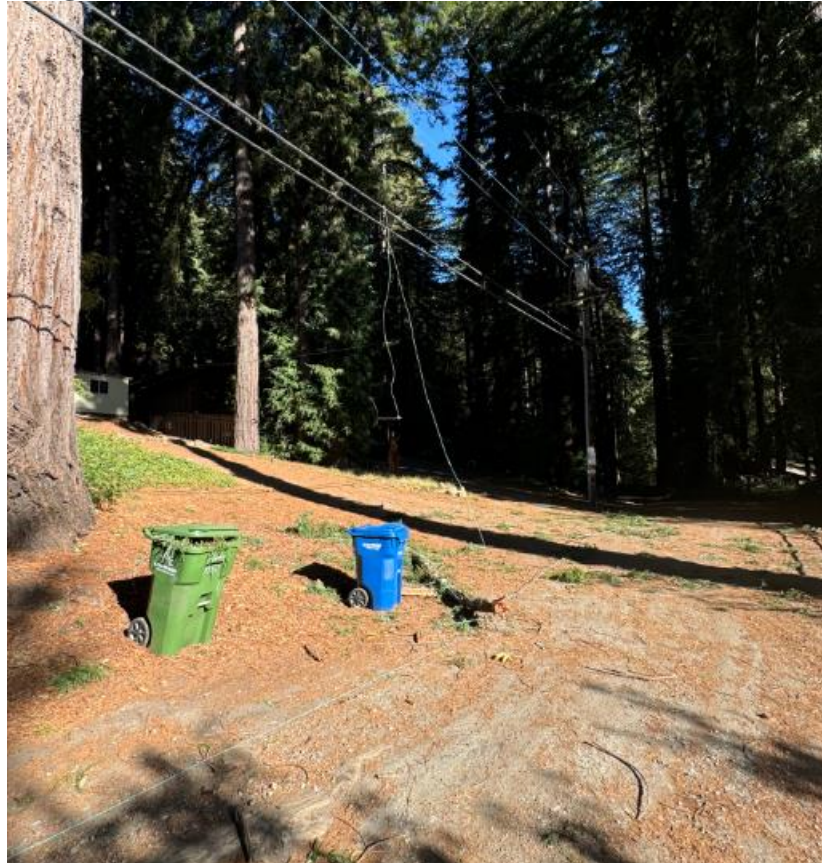
Figure 31: Vegetation-Damage in Santa Cruz County – Tree branch fell on wire
