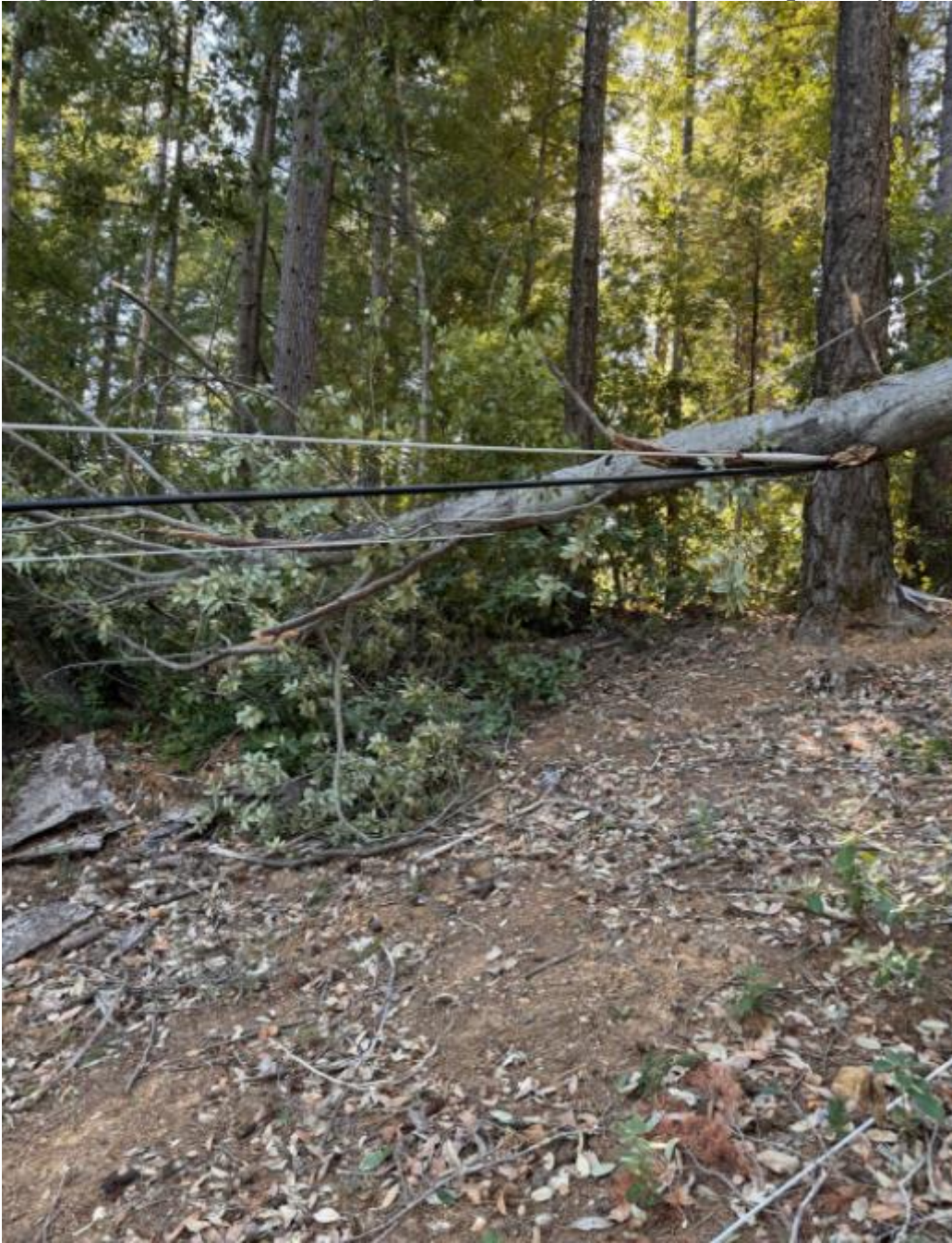
Figure 25: Vegetation-Damage in Napa County – Tree fell on primary line
