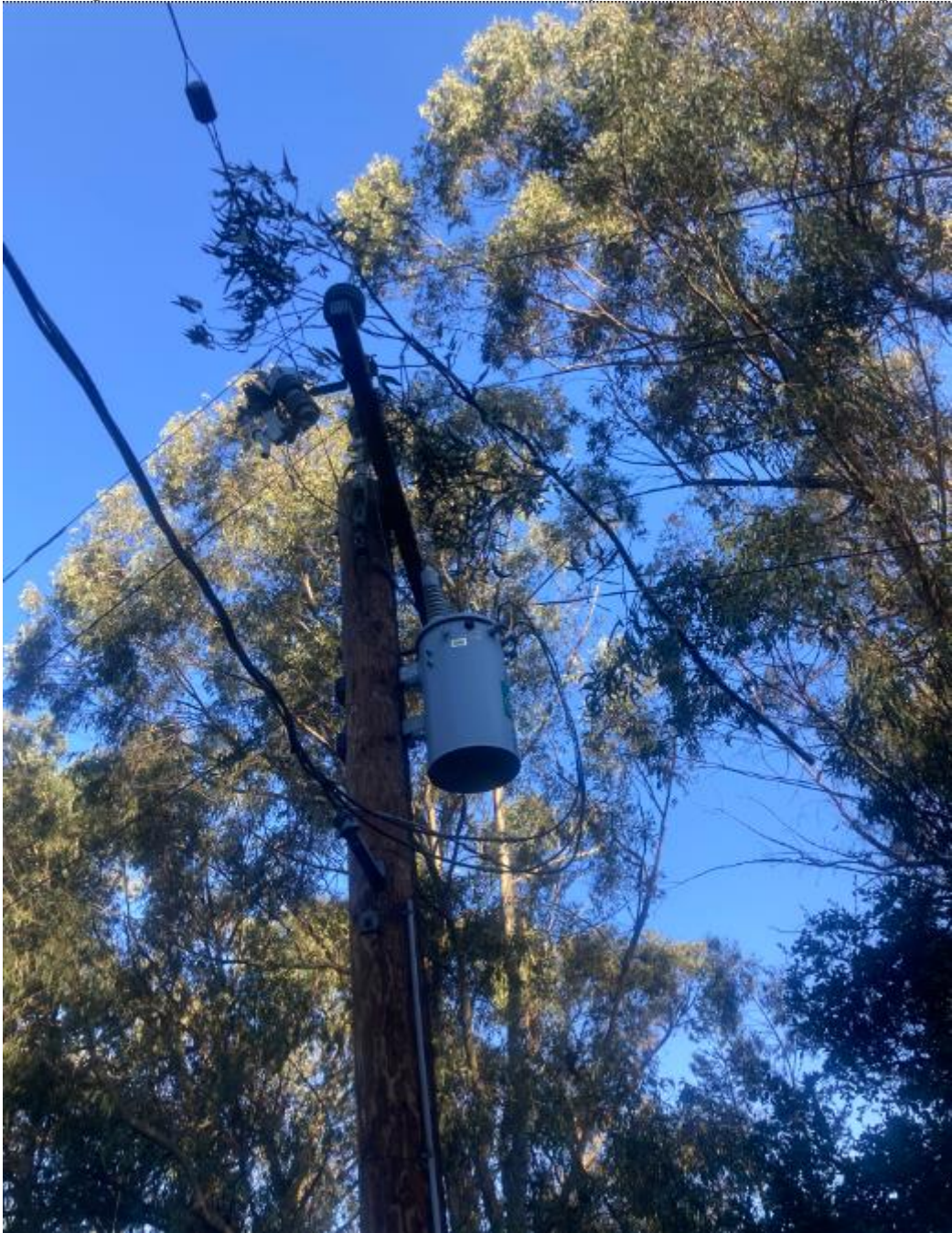
Figure 26: Vegetation-Hazard in Contra Costa County – Tree branch fell on primary line
