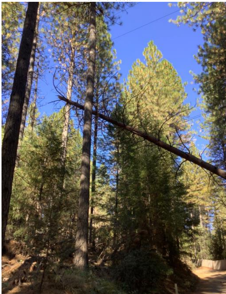
Figure 24: Vegetation-Damage in Butte County – Tree fell on primary line, broke pole top and crossarm
