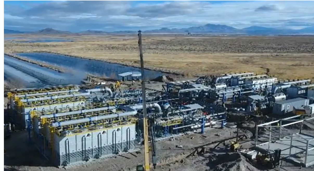
Open Mountain Energy's geothermal facility in NV
