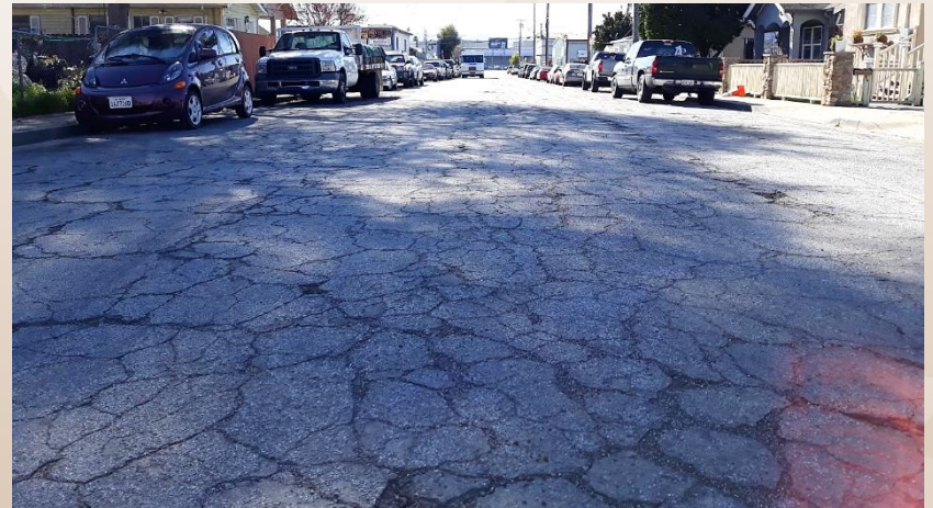
Santa Ana Ave: PCI 21, 1990 Chip Seal
