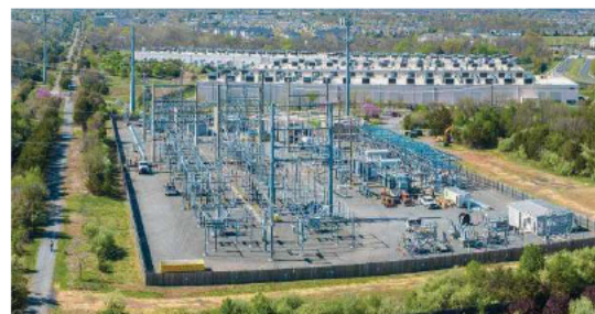
DC Substation Photo by Hugh Kenny/PEC
