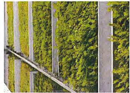
Fig. 4.12 Examples of techniques to mitigate blank walls - green walls, planted setback, public art, material changes, and lighting.
