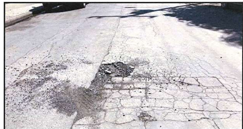
Failed (Below PCI 25) – Pacific Ave PCI 23
