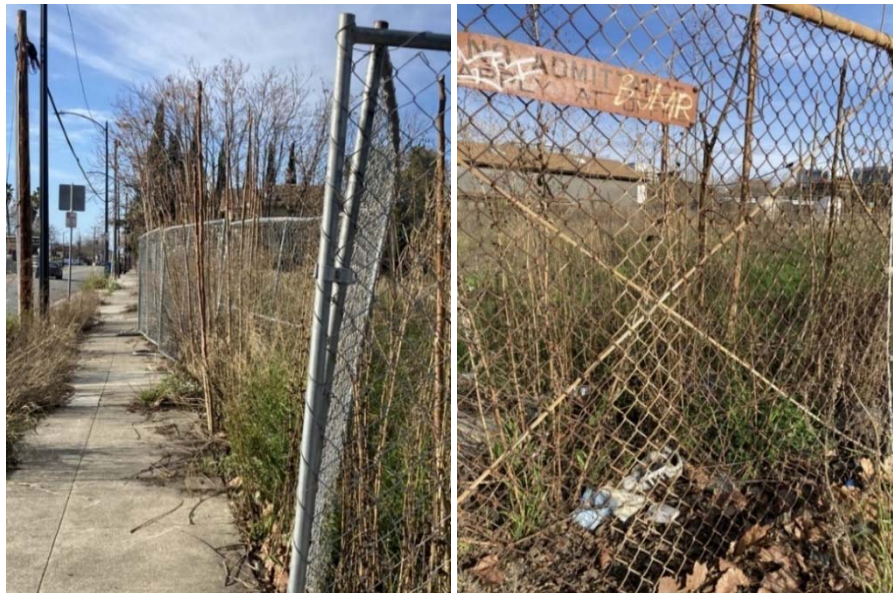
Source: Auditor photos of empty lot located behind the SAP Center, with overgrown weeds, broken fencing, and light graffiti.
