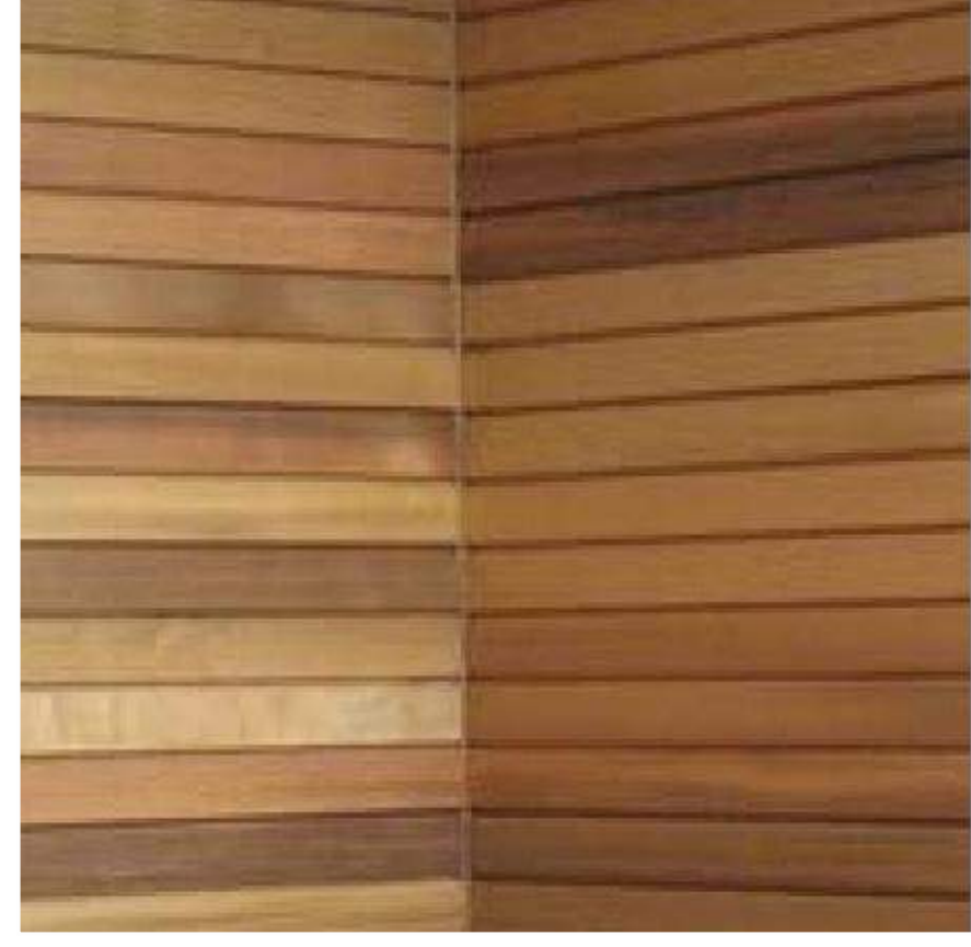
HORIZONTAL CEDAR SIDING Covers all exterior walls except where board formed concrete is specified as well as soffit
