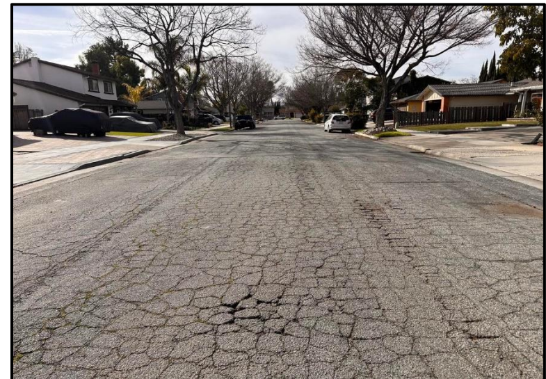
Failed (Below PCI 25) – Grandpark Cir: PCI 18
