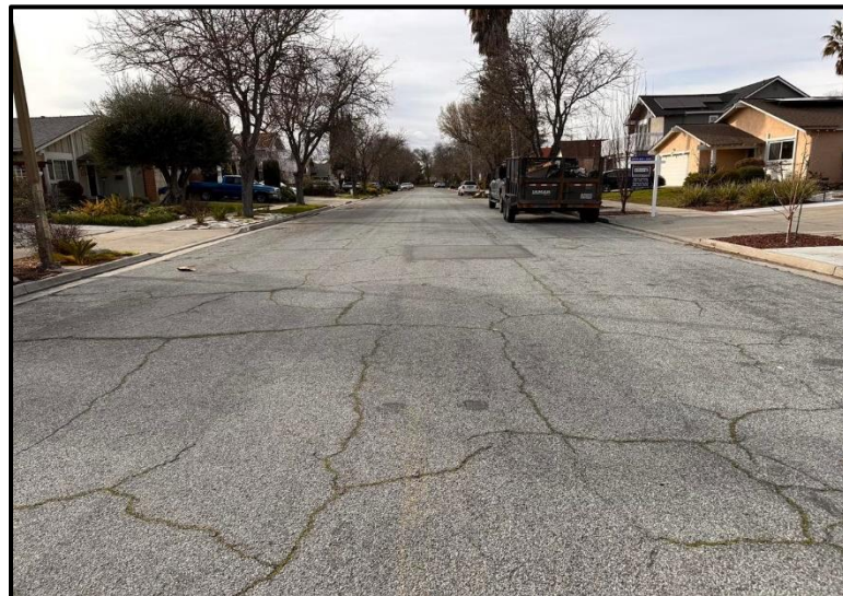
Poor (49 to 25) – Sposito Ct: PCI 39
