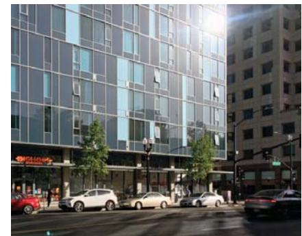
DO and DO NOT - Operable windows enhance livability and sustainability. Shading devices would have reduced the potential for glare.
