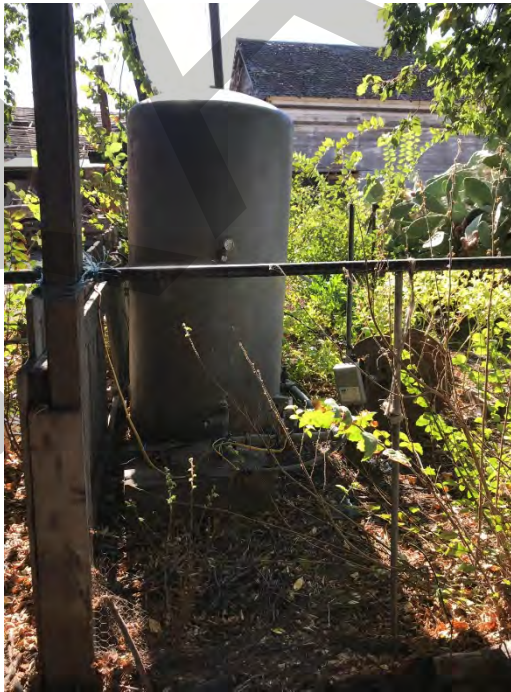
Southern portion of the Emado Compound. Residential well located to the north of the western single-family residence (also shown in Photograph 71).
