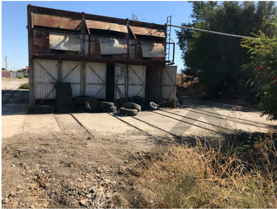
Northern portion of the Emado Compound. Tires, bikes, and other debris on north side of cinder block building.
