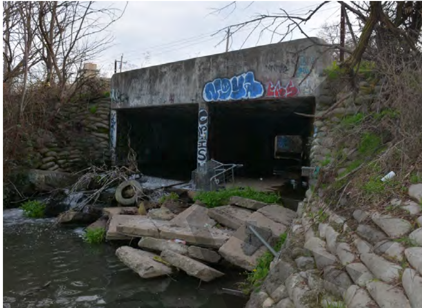
Fisher Creek culvert under Monterey Road. Photo by Pathways for Wildlife.
