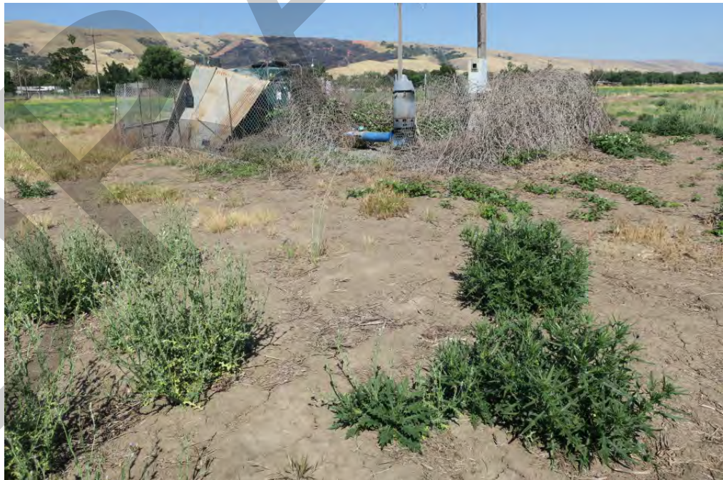
Well and associated water infrastructure including water tank and electricity drop near the center of the Fisher Flats parcel 708-25-004, showing ruderal vegetation around the well.
