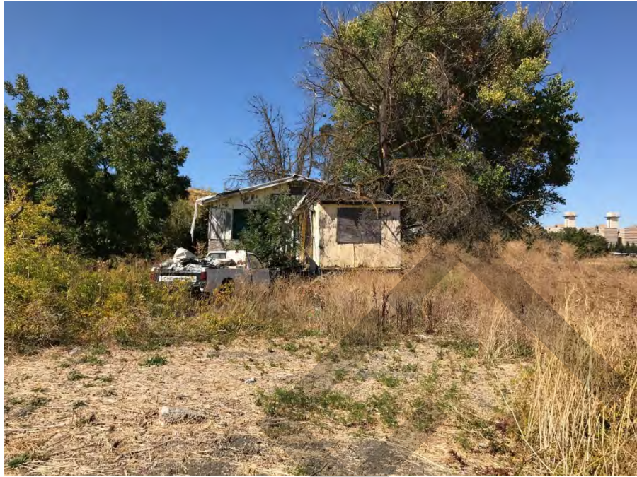
Back of single-family home in Blanchard Residential Area; to be demolished. Pick up truck full of debris.
