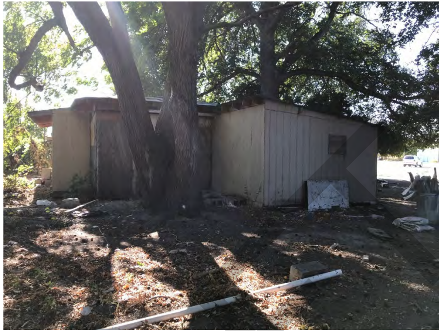
Southern portion of the Emado Compound. Eastern side of western single-family residence.
