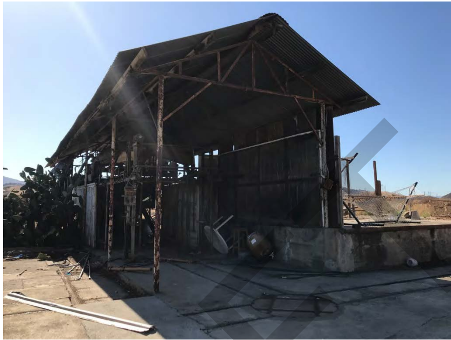
Southern portion of the Emado Compound. Southern side of the tin roofed pole barn.
