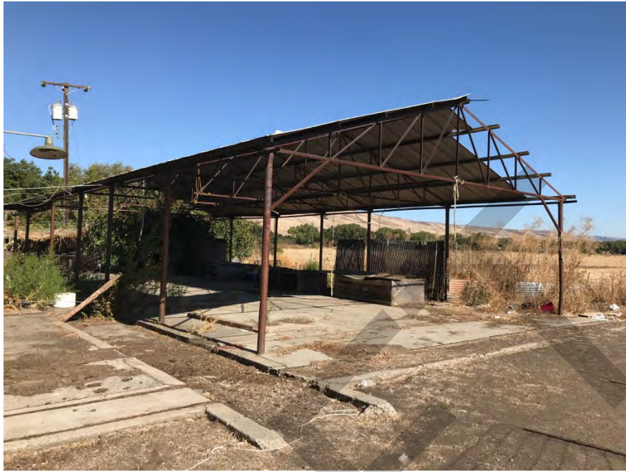
Southern portion of the Emado Compound. Second tin roofed pole barn south of eastern cinder block building with concrete pad with missing portions of the roof.
