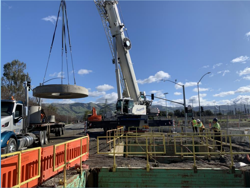
Large Trash Capture Installation Quimby Location February 2024
